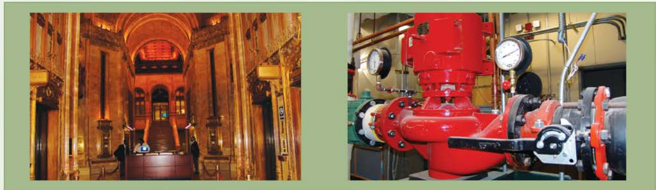
Woolworth Building —EnviroFlo Close-Coupled Vertical In-Line Pumps are providing worldclass quality and reliability as they circulate condenser water to 18 units on three floors of this world-renowned structure in NYC.
